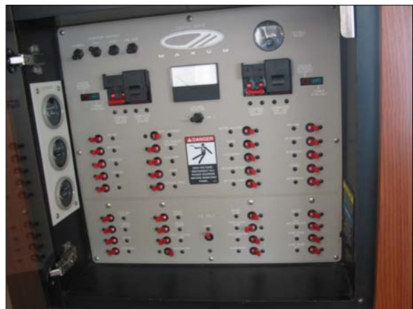
AC/DC power distribution panel
