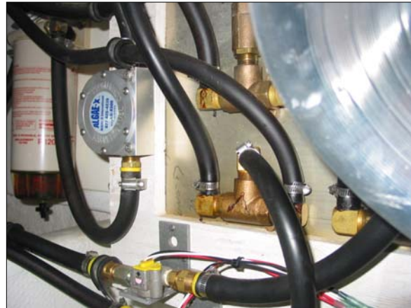
Fuel shut off valve, Racor filter and Algae-X system
