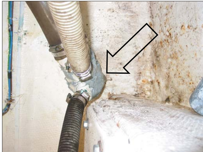
Log port cockpit drain with putty repairs
